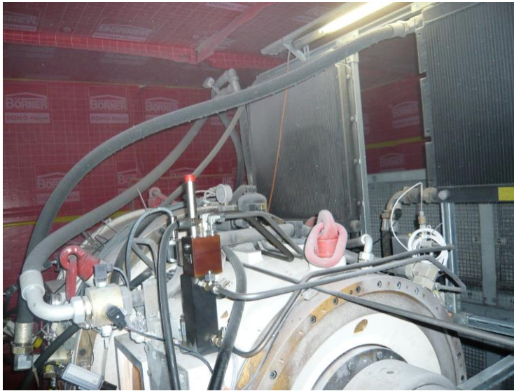
Picture 2: WinDrive and coolers at -35 °C (-31°F)
